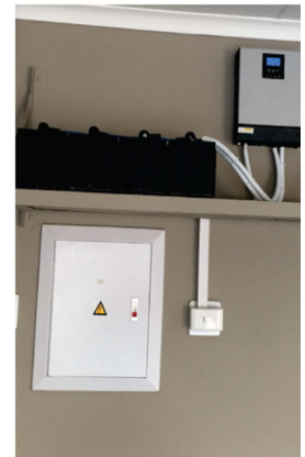
3kVA Inverter installed on shelf above main DB
