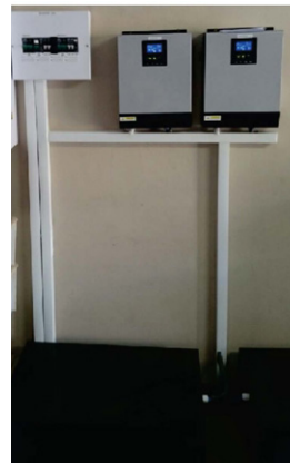
Dual 3kVA Inverter installation with Sb-DB
