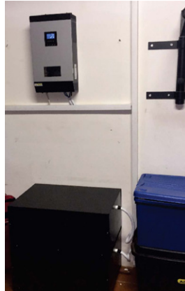
5kVA Inverter in home garage with dual battery cabinets
