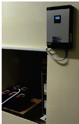
5kVA Inverter with SB DB for dedicated circuits
